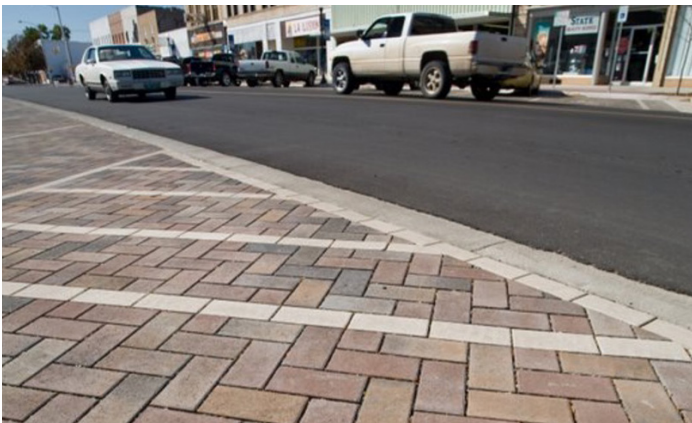
Photograph PPS-3. PICP in downtown Ft. Morgan, CO. Note soldier course of light-colored pavers where PICP meets conventional pavement. Photo: SEH and the City of Ft. Morgan.
