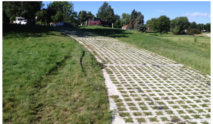
Photograph PPS-6. Reinforced grass pavement using concrete grid for maintenance access to a stormwater pond.
