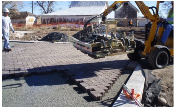
Photograph PPS-20. Mechanical placement in larger areas can reduce the unit cost of the pavement. Photo: Muller Engineering Company and Jefferson County Open Space.
