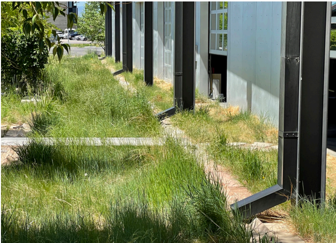
Photograph 4-14. Disconnected downspouts discharge to grass swale to dissipate concentrated flows and allow for infiltration and filtration. Vegetation provides energy dissipation.
