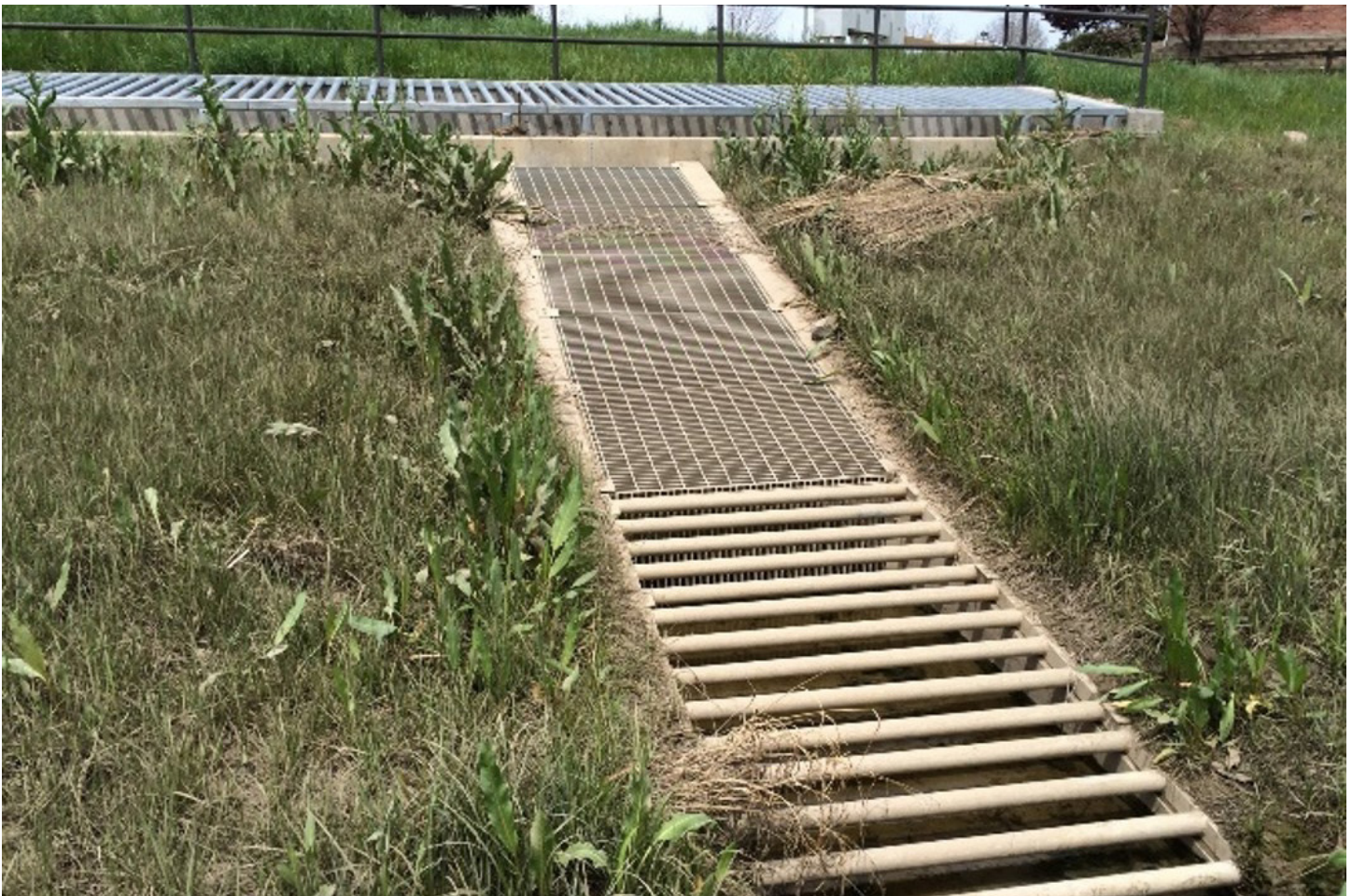
Photograph EDB-3. Outlet structure with coarse safety grating covering the micropool in the foreground, standard bar grating flush with the top of parallel concrete wingwalls and extending down through the micropool, and coarse safety grating covering the 100-year drop box in the background.
