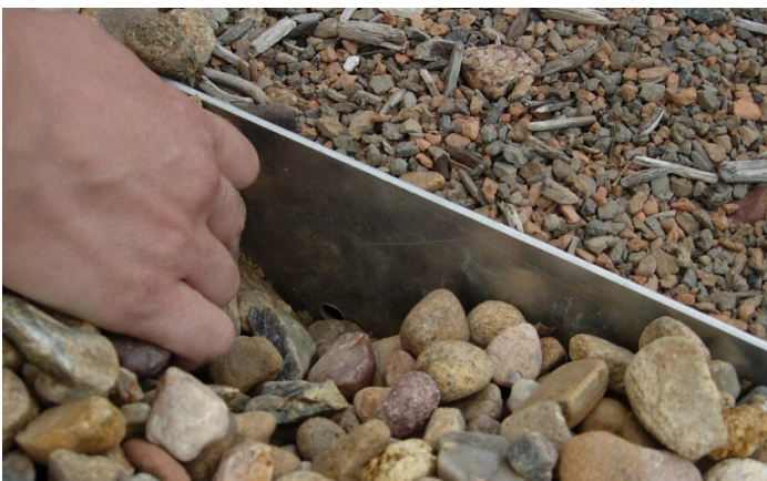
Photograph GR-4. The metal edging has perforations near the bottom to allow flow into the drain.
