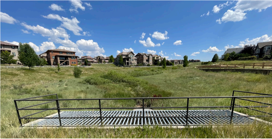
Photograph EDB-2. This EDB depicts a meandering low flow channel with adjacent benches that remain drier to allow equipment access for maintenance.
