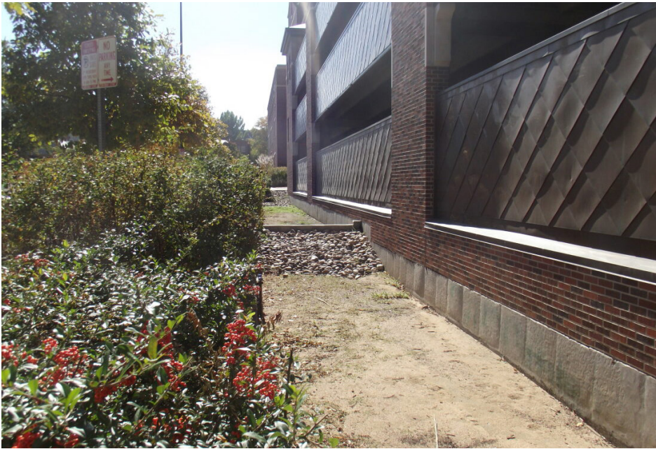
Photograph SF-1. This sand filter, constructed on two sides of a parking garage, is accessible for maintenance, yet screened from public view by a landscape buffer.
