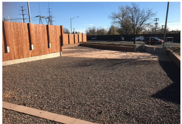
Photograph SF-3. Sand filter with incorporation of minor event flood attenuation provides water quality and detention for a substation.
