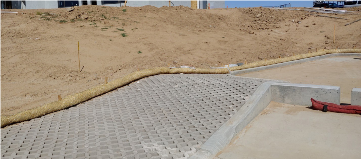
Photograph PPS-18. Concrete cellular paving grid for RGP provides maintenance access to the forebay. Photo: Creative Civil.
