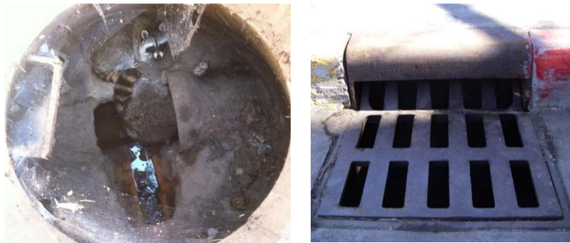
Raccoons inhabiting storm sewer system (a) and retrofitted storm drain inlet (b). (Photos courtesy of Andy Taylor, City of Boulder, CO)
