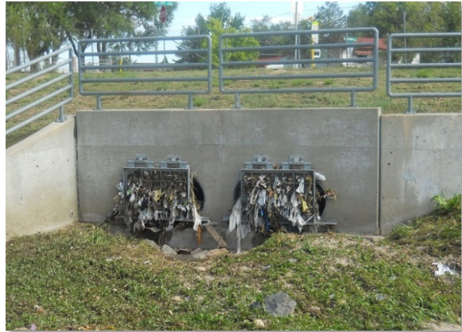
Photograph 11-3. Grating at conduit outlets are prone to clogging and will hamper rescue efforts, cause pressurization of the pipe, and potentially flood upstream areas.
