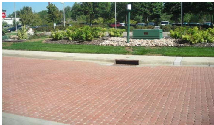
Photograph 1. PICP with sampler box and rain gauge shown in background.
