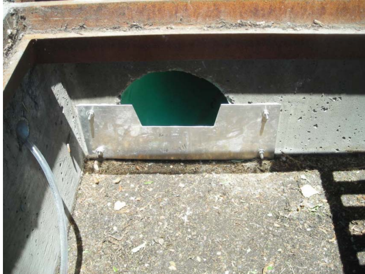
Photograph 6. The inlet of the reference site, shown with Cipoletti weir
