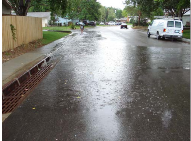
Photograph 7-6. Weir performance decay can be observed in this picture as flow appears to enter only the first two inlets while exceeding the height of the upstream curb.
