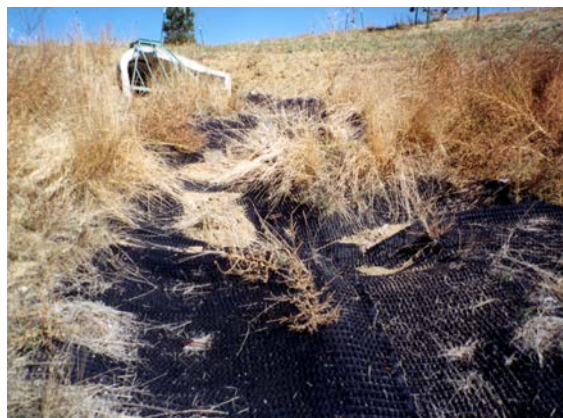
Photograph 9-28. Pipe outfalls are recommended over rundowns due to the high failure rate of rundowns.
