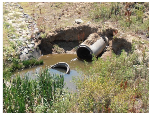
Photograph 9-29. Pipe end failure resulting in loss of the flared end section
