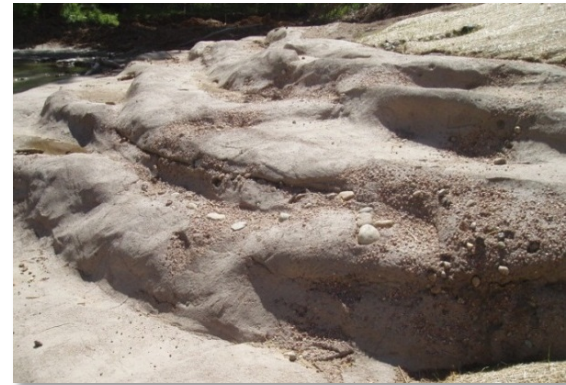
Photograph 9-16. Completed sculpted concrete drop structure with loose sand, gravel and cobble embedded into the surface.
