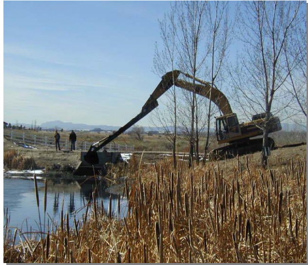
Photograph 6-1. Sediment removal from a forebay at the regional Shop Creek BMP System.
