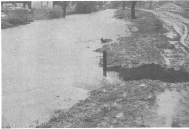
Breach near South Quebec Street and East Evans Avenue
