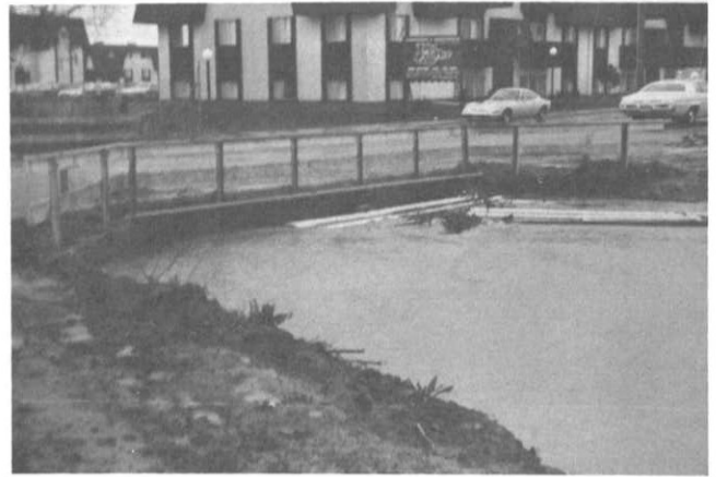
Highline Canal near breach on South Quebec Street
