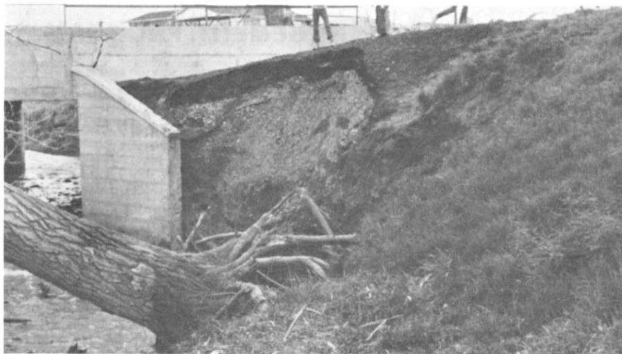
An example of the type of problems requiring maintenance
