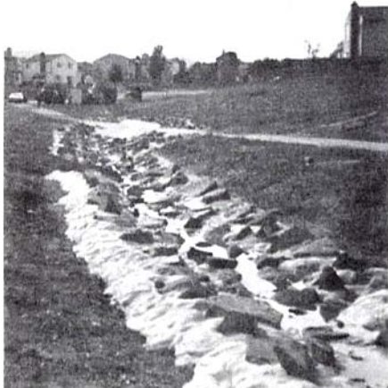
Lake Park drainageway at Griffith and Lincoln in Louisville. This is a trapezoidal grouted riprap channel.
