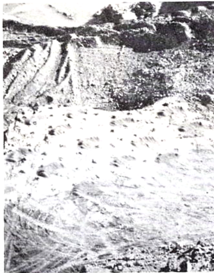
Figure 1 - Looking down on a rock ledge that has been drilled, had explosives inserted and is ready for blasting.
