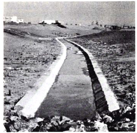
Lone Tree Creek south of Arapahoe Road. This is a trapezoidal concrete channel.
