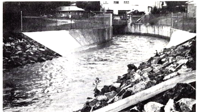
Figure 9 - Riprap used in a transition from a concrete lined channel to a grass lined channel.
