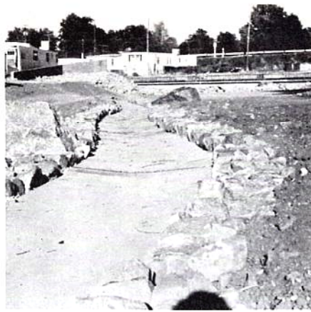
Little's Creek south of Bowles and west of Santa Fe in Littleton. This channel has a concrete bottom with rock sides which results in a pleasing appearance.
