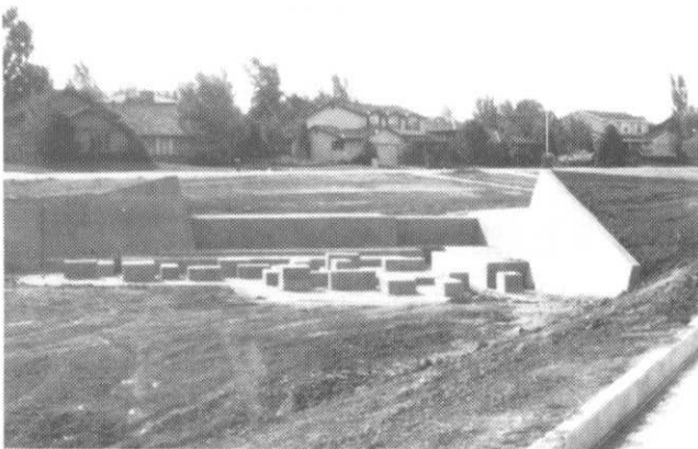
Drop structure on Goldsmith Gulch. Note trickle channel on the side of the pond.
