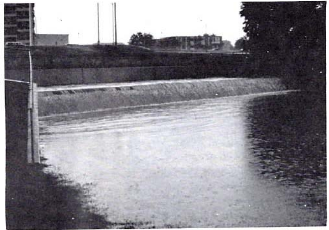
The side channel spillway into the off-line detention at Veterans Park in Denver on July 20, 1991.
