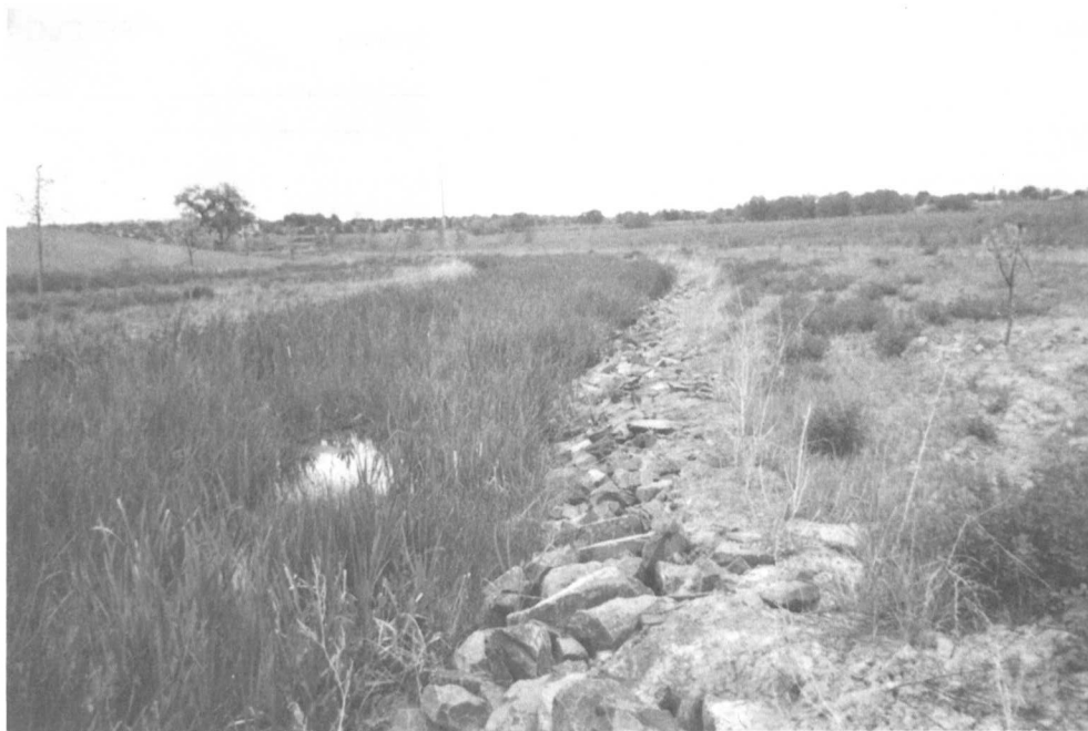
A wetland bottom channel on Walnut Creek in Westminster designed according to the Urban Storm Drainage Criteria Manual within one year of completion.
