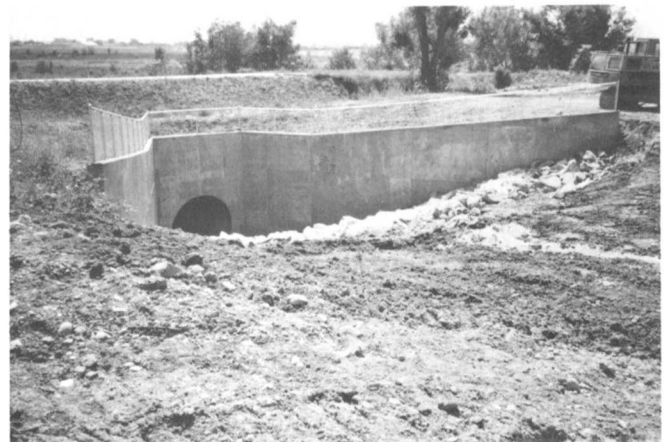
Kalcevik Gulch flow separation structure.
