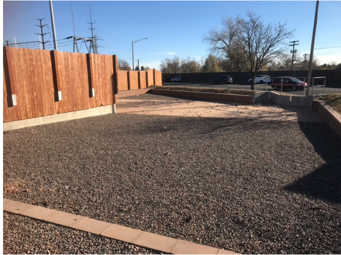
Photograph SF-3. Sand filter with incorporation of minor event flood attenuation provides water quality and detention for a substation.
