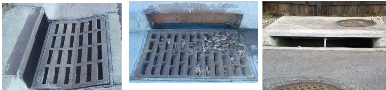
(a) CDOT Type 13 grated inlet in combination configuration
