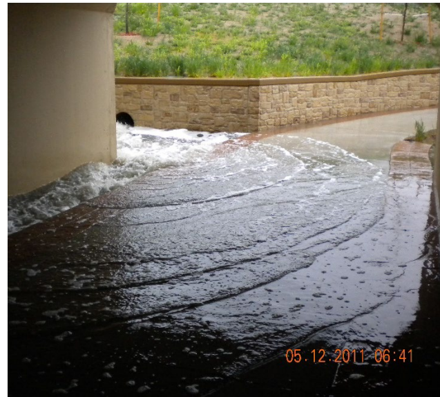
Tommy Davis Park detention outlet (on north side of berm in underpass) looking south.
