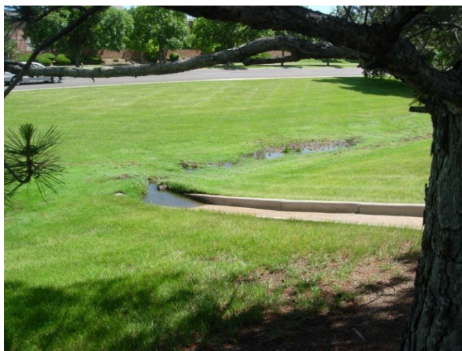
Photograph 6-2. A lack of sediment removal in this grass swale has resulted in a grade change due to growth over the deposition and ponding upstream.
