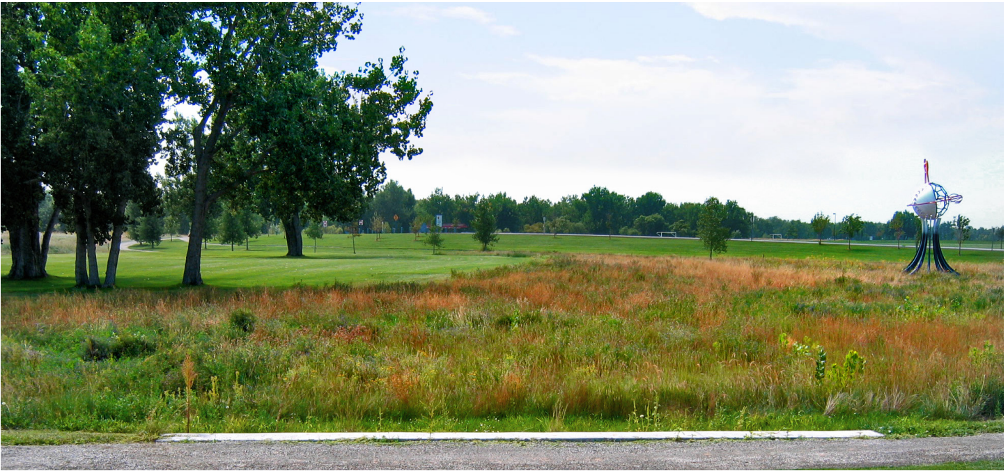
Photograph 4-13. Level spreader at Aurora Sports Park evenly spreads flow to the wetland area downstream.
