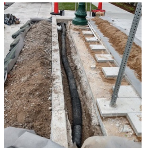
Photograph PPS-7. Perimeter barrier and trench with underdrain to protect street subgrade with adjacent PPS installation. Photo: Beck Group.
