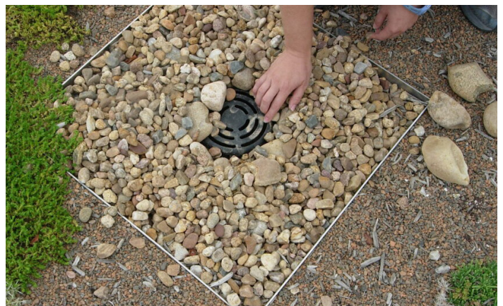
Photograph GR-5. Metal edging separates substrate from rock that surrounds the roof drain. It also serves to facilitate regular maintenance by limiting plant and root growth near the drain.
