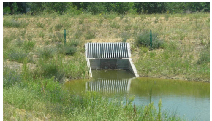
Photograph 4-18. Although each site is different, most sedimentation SCMs have similar outlet structures. Each structure should include a partially submerged orifice plate with a screen (or grate) protecting the orifice plate from clogging, and an overflow weir for flows exceeding the WQCV or EURV when full spectrum detention is used.
