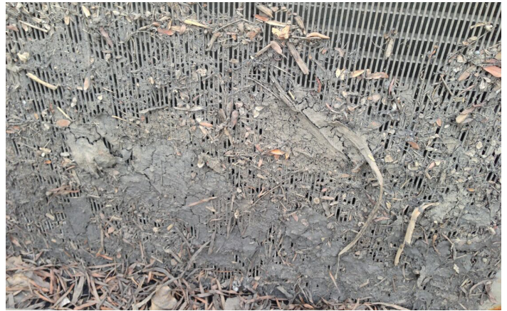
Photograph EDB-5. Well screen is intended to protect small orifices from clogging; however, the fine screen is itself subject to clogging and requires frequent inspection and maintenance to keep clear.
