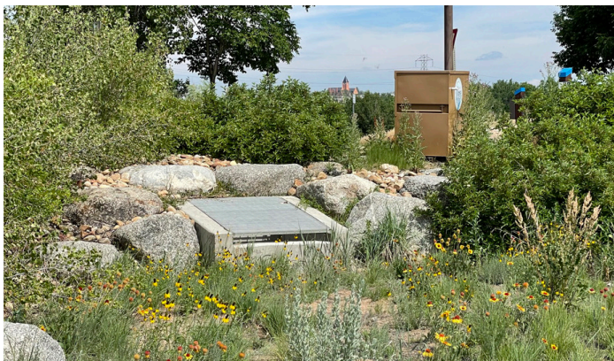
Photograph 4-17. Outlet for bioretention system at River Run Park. The WQCV is filtered through media and infiltrates or discharges to the outlet via an underdrain. The outlet is also designed for detention of larger events with a weir control (i.e., top of outlet box) overflow. The spillway for the basin is provided as a low spot above the outlet near the rain gage.
