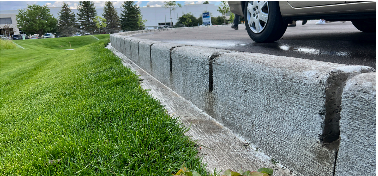
Photograph 4-8. Typical slotted curb showing drop from slot to adjacent pervious area to allow for growth of vegetation and sediment accumulation. This area provides for mowing and maintenance access to keep positive drainage from the parking lot to the RPA.
