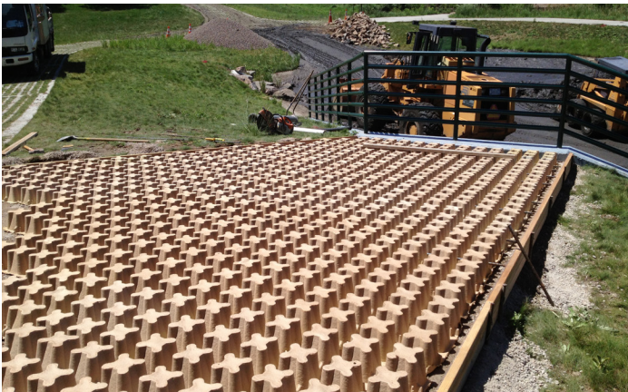
Photograph PPS-16. Forms for concrete grid for reinforced grass pavement to access pond outlet structure.
