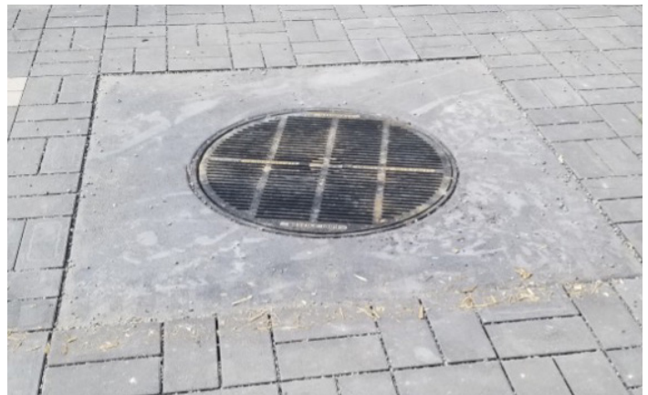
Photograph PPS-15. Concrete collar helps avoid small-cut pavers around edges of inset features and can be colored to match surrounding pavers. Photo: Creative Civil.
