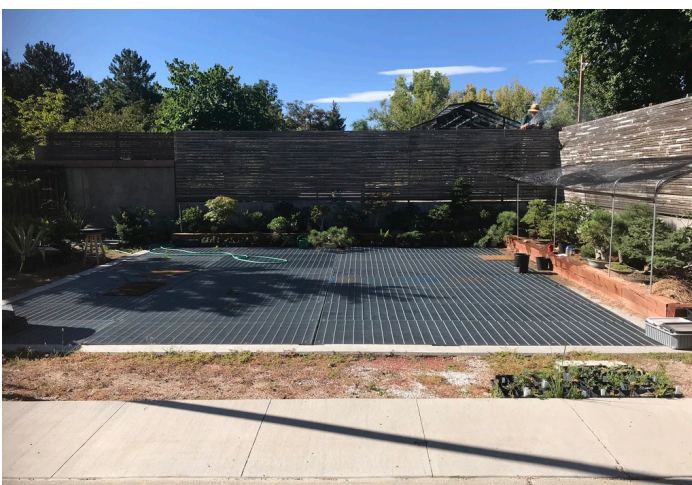
Photograph SF-2. Underground sand filter at Denver Botanic Gardens has a grated top, which enables inspection and maintenance.
