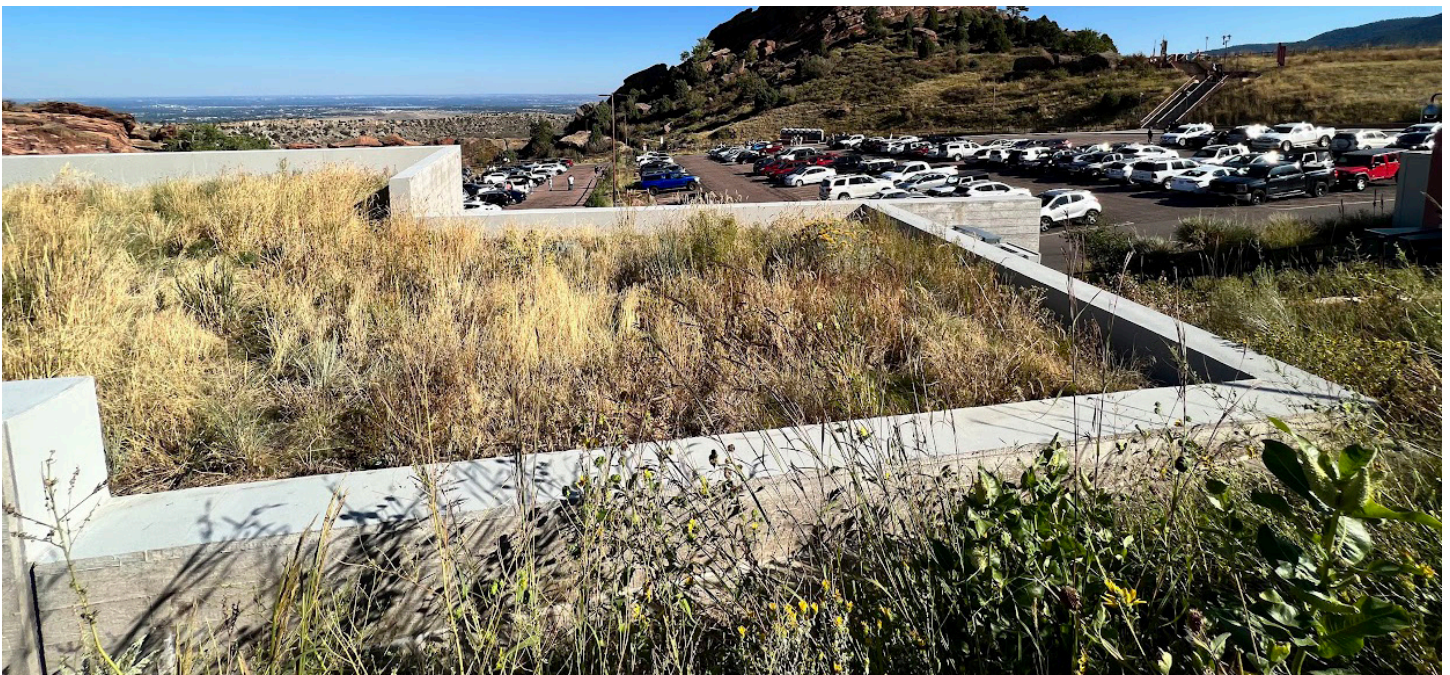
Photograph GR-6. A green roof installed on a maintenance and restroom building at Red Rocks Park and Amphitheatre promotes sustainable design and adds aesthetic value.
