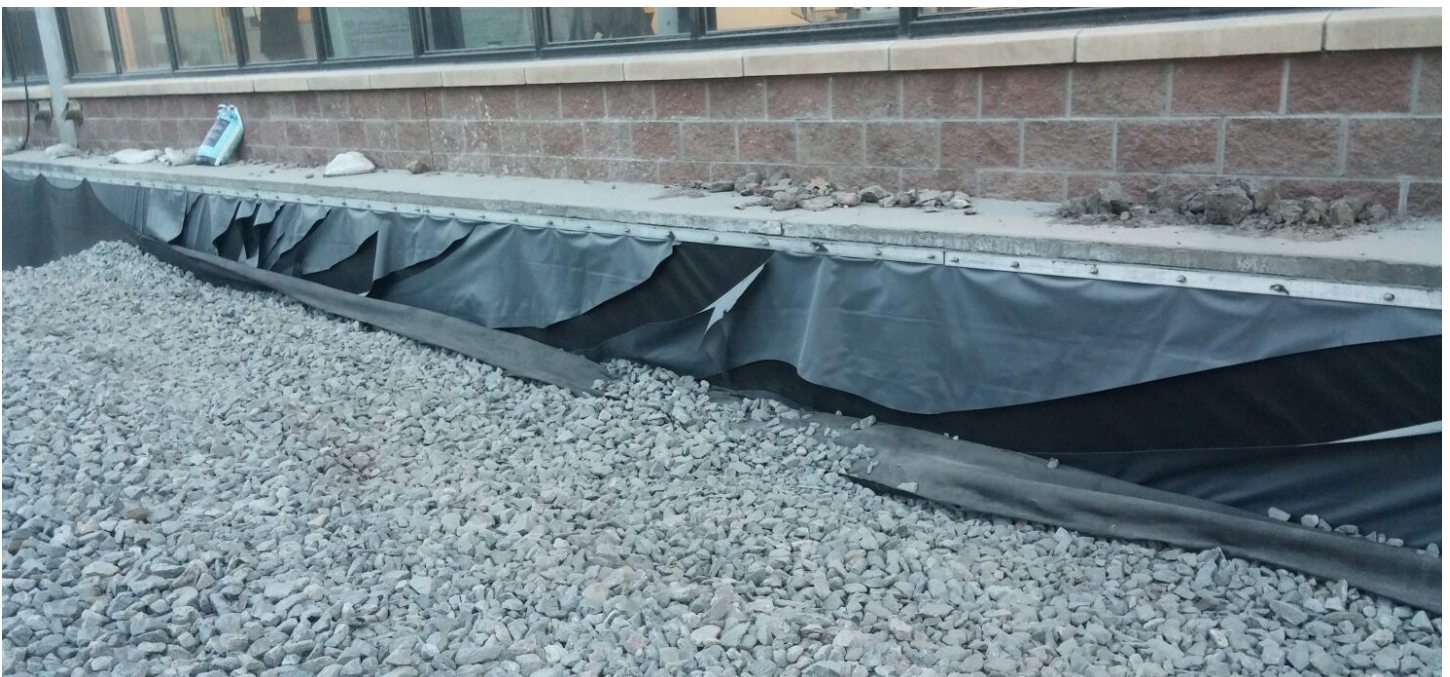
Photograph 4-5. Liner tear after aggregate placement (even with slack provided). To avoid this problem, delay attaching the liner to the perimeter barrier with a batten bar until after placing aggregate by temporarily anchoring the liner.
