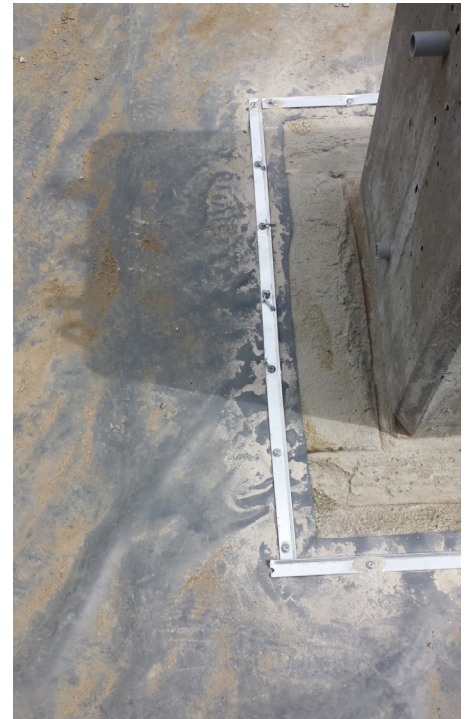
Photograph PPS-11. Geomembrane attachment to horizontal footing for light pole. Photo: Creative Civil.
