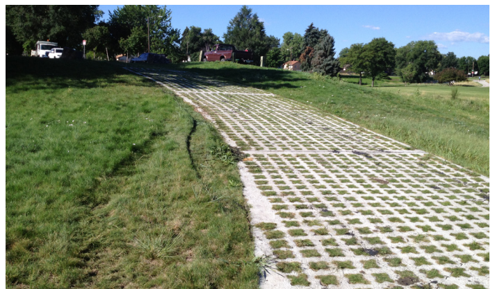
Photograph PPS-6. Reinforced grass pavement using concrete grid for maintenance access to a stormwater pond.
