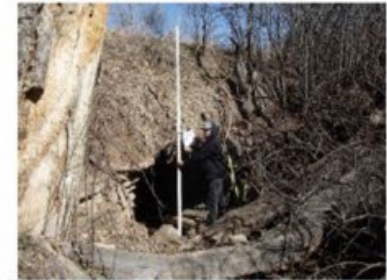
Reach WC-5: Structure 21 – Belleview Avenue (1) 78-inch CMP
