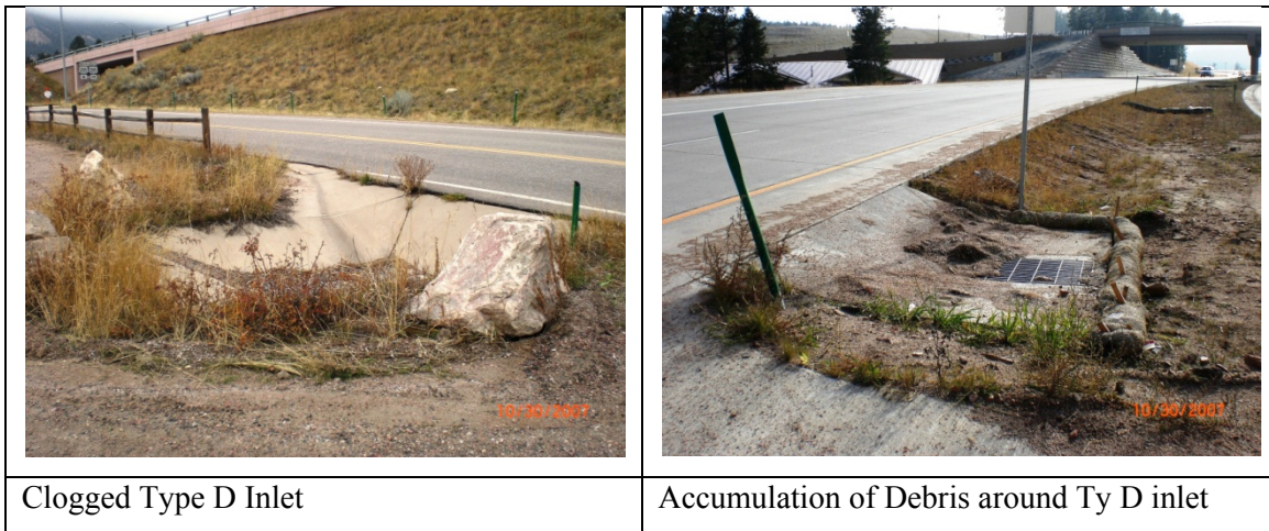
Figure 13 Clogging Condition around Type D Inlet in Field
